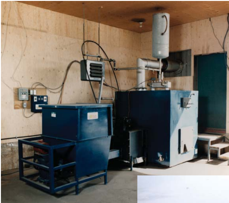
Power Line Pork, Borden, Prince Edward Island Facility Type: Pig farrowing farm System Size: 1 MMBH (two-boiler) Manufacturer: Grove Wood Heat Heating plant is housed in shed on left (lower photo). Fuel is delivered to overhead door and pushed onto shed's floor slab for storage, using tractor. Two side-by-side "Bioblast" systems (like the one in photo at left), located in the same shed, are sized at 45% and 55% of peak load. Each Bioblast consists of a tractor-loaded day bin (shown in foreground), a combustor (middle) and a boiler (rear).
