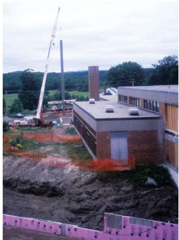
Union 32 Junior-High School, East Montpelier, Vermont. 4.5MMBH Manufacturer: Messersmith Manufacturing Installation of a tall stack.
