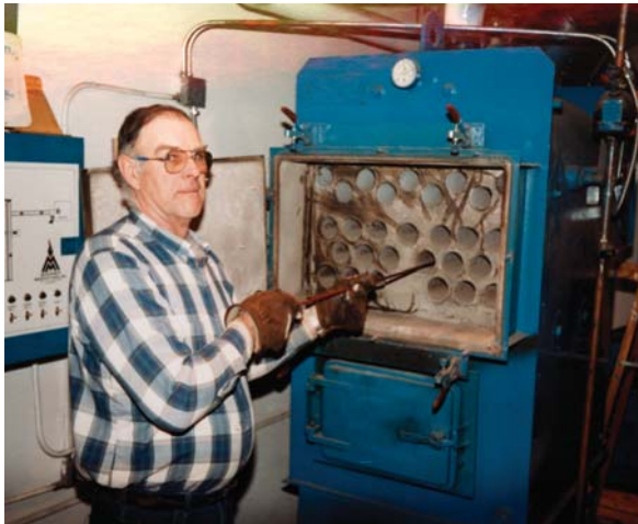
Boiler Tube Cleaning Manual boiler tube cleaning shown at Calais Elementary School, Calais, Vermont (.5 MMBH system by Messersmith Manufacturing).
